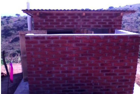
Fig 1: Kunenekude maternity unit bathroom and toilet
